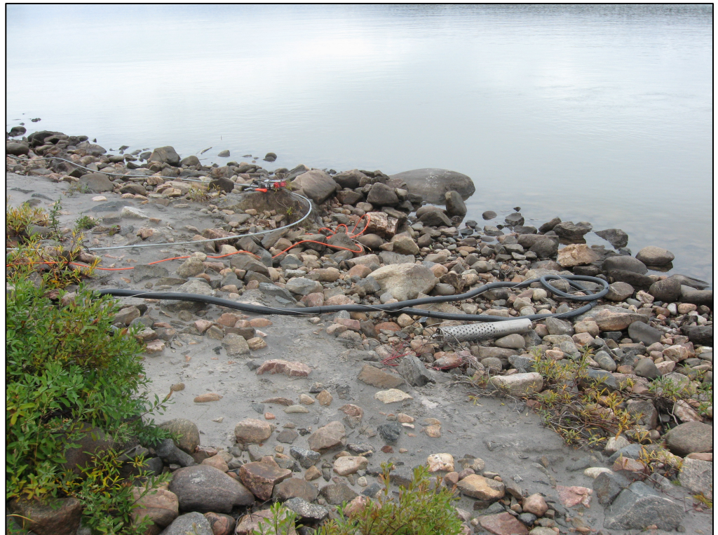
Figure A-2: Photograph of protective electrical conduit that houses the cable connecting the Datasonde to the hut. Also visible is the cylindrical metal casing where the Datasonde is located during deployment.
